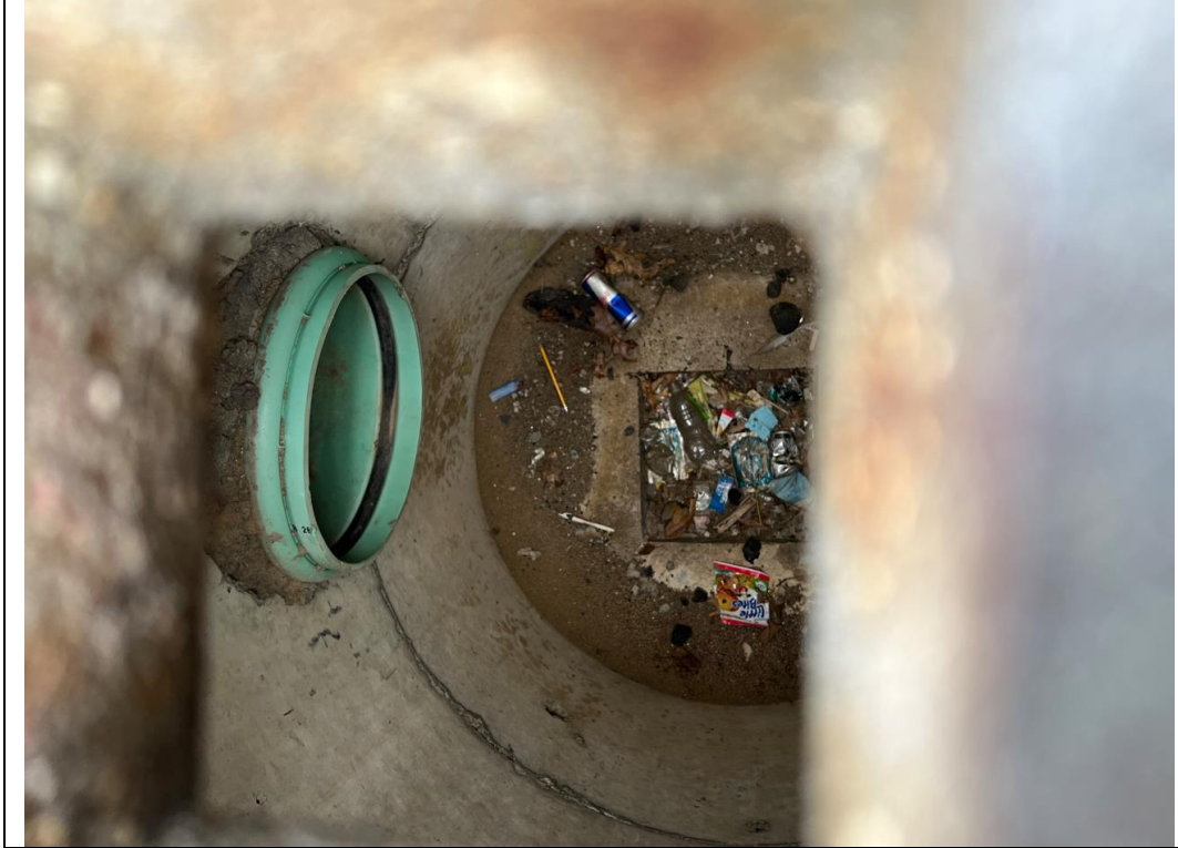
Figure 23: Catch basin with some debris and sediment.
