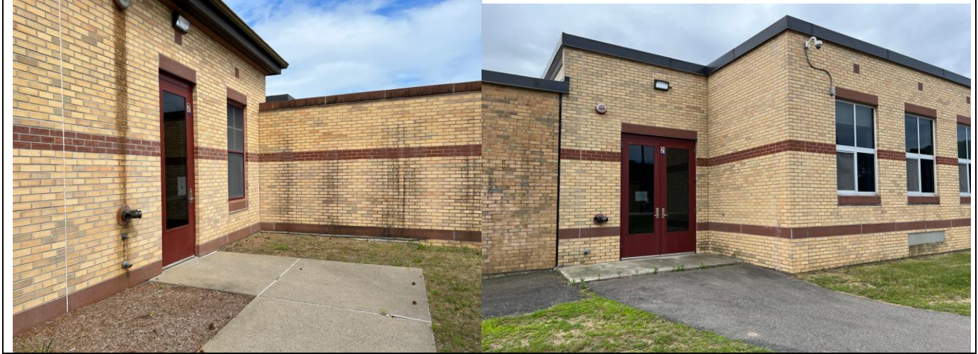
Figure 26: Southeastern FD connection and north FD connection.
