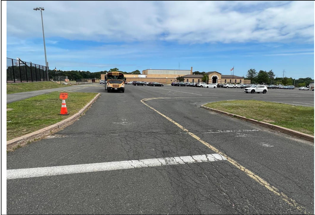
Figure 03: Typical condition of asphalt pavement on the campus, with alligator cracking visible.
