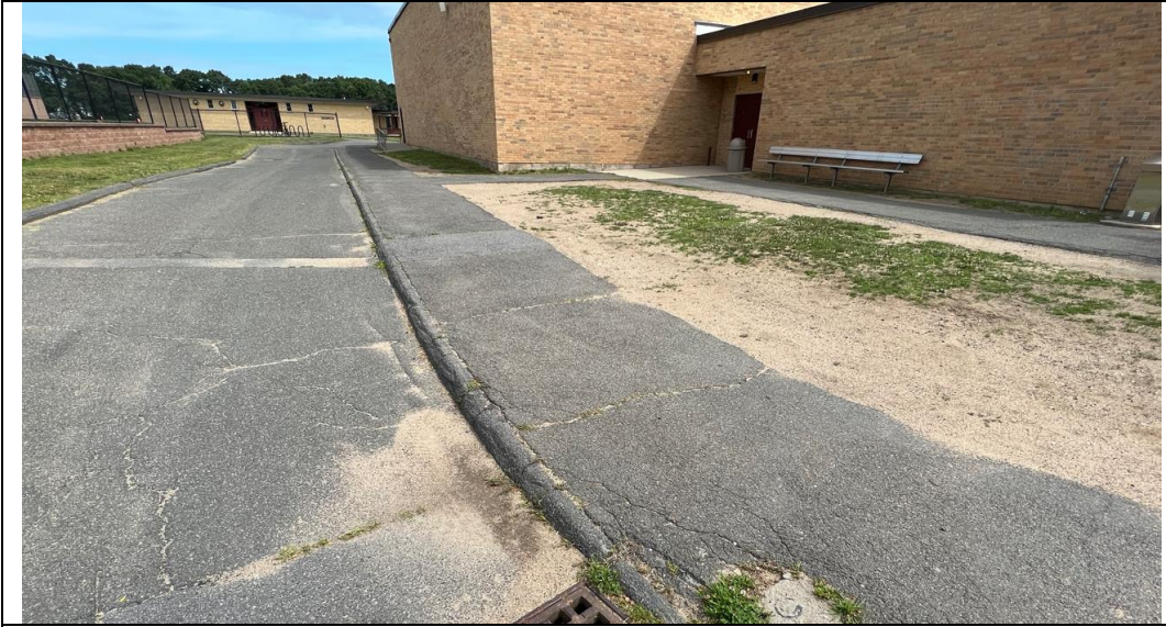
Figure 07: Typical condition of bituminous asphalt walkway on the campus.
