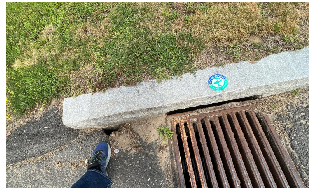
Figure 22: Small sinkhole observed at granite curb next to catch basin.
