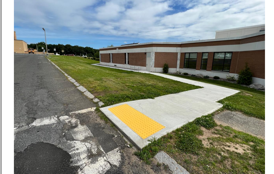
Figure 09: ADA/MAAB non-compliant crosswalk and curb ramps at the library across from the existing high school. The new ADA access should integrate with that existing ADA ramp.
