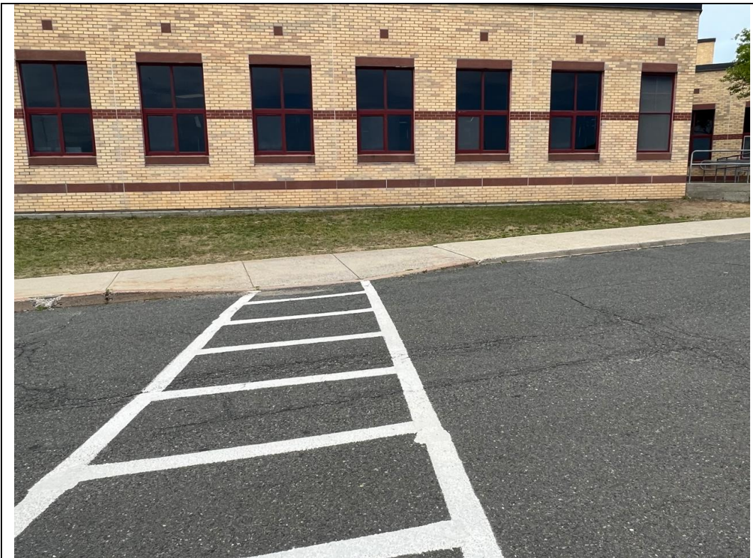
Figure 12: ADA/MAAB non-compliant crosswalk and curb ramps.
