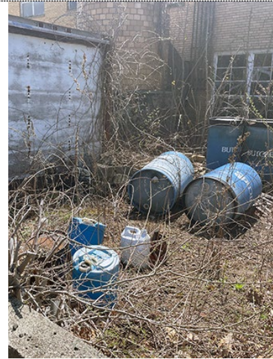
Image: Various building and maintenance materials are stored uncovered in a courtyard space.
