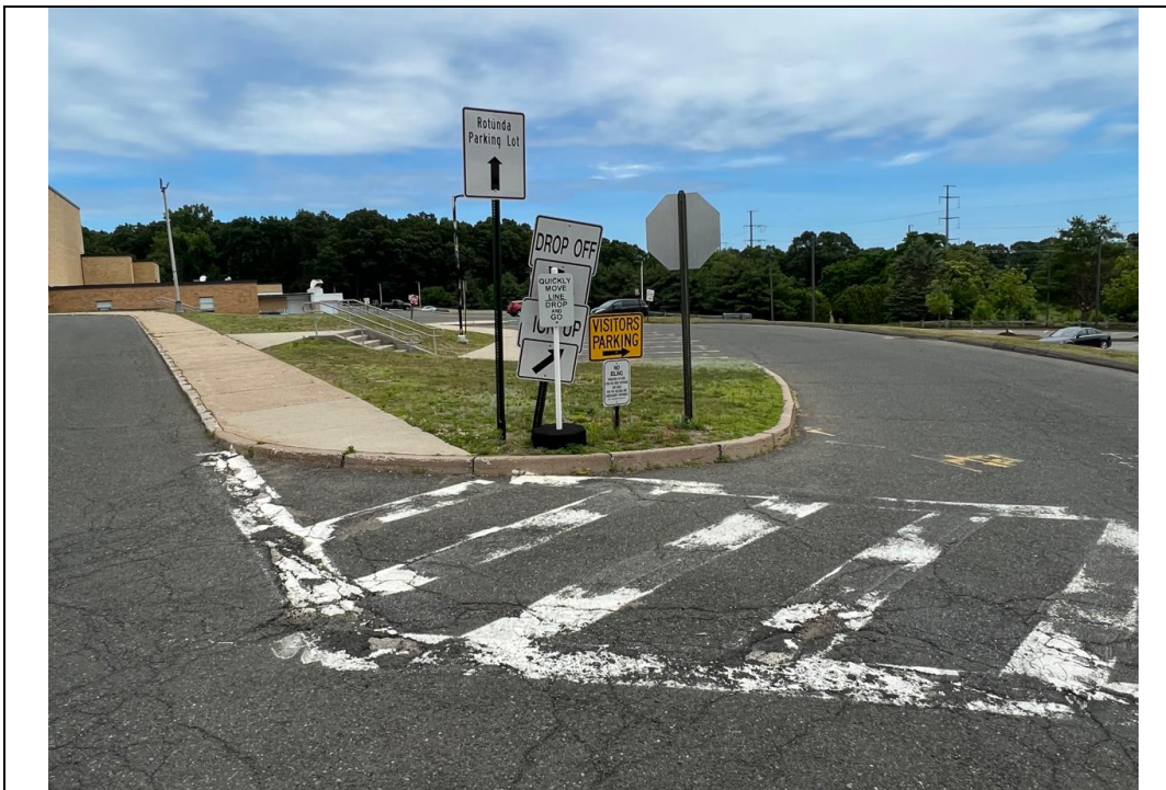
Figure 10: ADA/MAAB non-compliant crosswalk and curb ramps.
