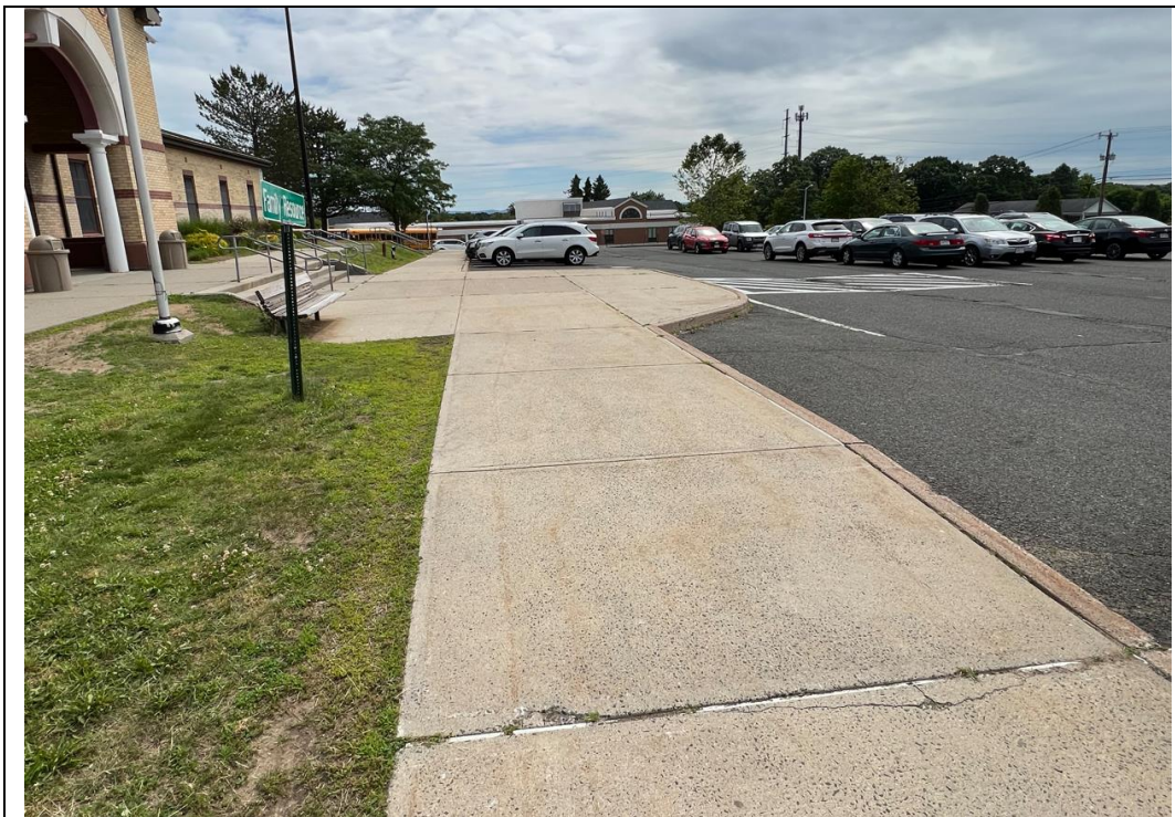
Figure 06: Typical condition of concrete walkways on the campus. Accessible curb cut needed at crosswalk stripping.
