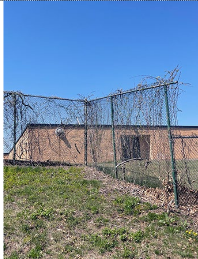
Image: Chain link fence in poor condition near the northeast corner of the school.
