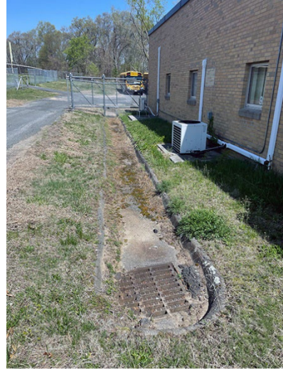
Image: Asphalt drainage swale encumbered by moss and grasses.
