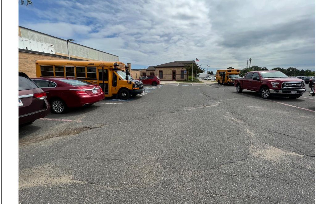
Figure 05: Longitudinal (Linear) and transverse cracking of bituminous paving in primary parking Lot.
