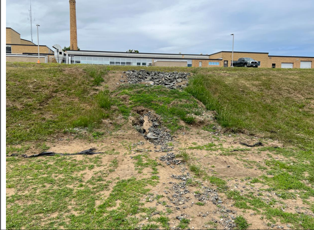
Figure 25: Rip rap at main DCB in the rear parking area, with debris and sediment noted. This area has clearly been a major erosion point and should be addressed with improved drainage infrastructure.
