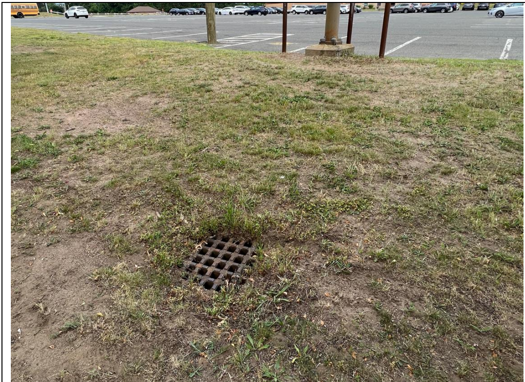
Figure 24: Overgrown catch basin drainage cover.
