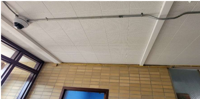
Camera Cables in Conduit (Data cables in surface mounted raceway and exposed)
