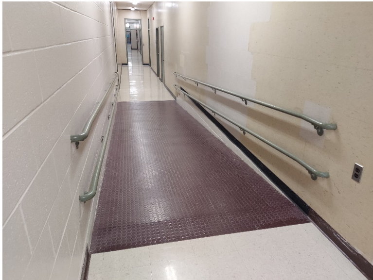
Lower Level Ramp w/ Slope that Exceeds 8.3%
