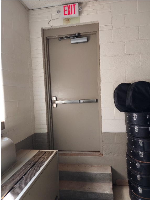
Music Room Egress Stair without Handrails
