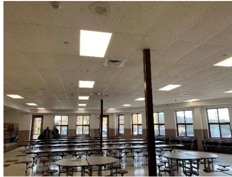
Cafeteria expansion with ducted supply grilles
