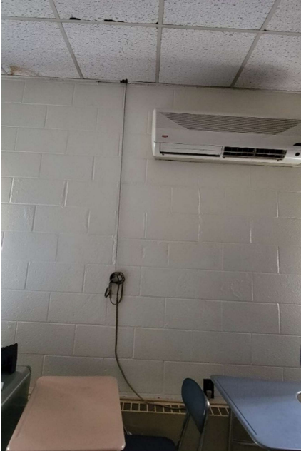
IDF in Town Building Room (IDF is a Network Switch above the ceiling resting on T-rail)
