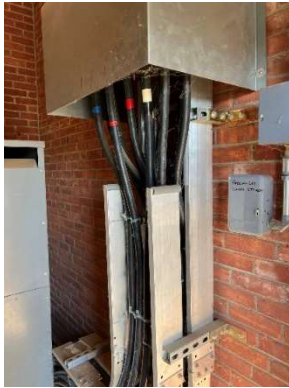
Backfeed to Original Service
