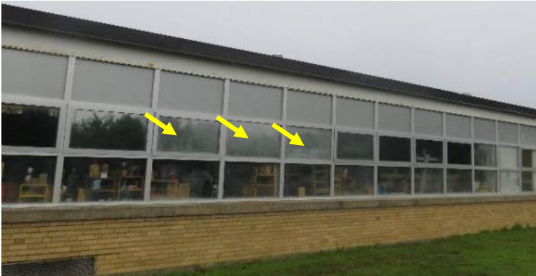
Arrows identify failed glazing seals. Note the metal faced transom panels above the windows.
