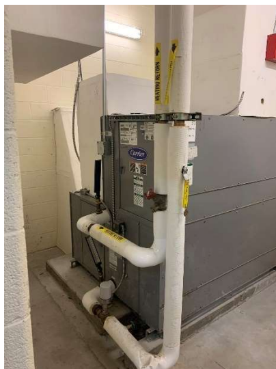
Mid-1990's cafeteria expansion Carrier AHU
