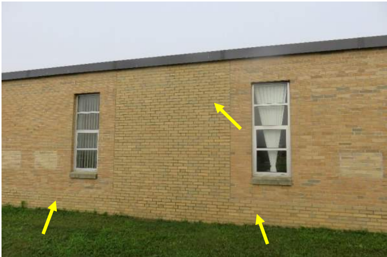
Perspective view of 1955 wall construction with subsequent modifications made thereto in 1979 with the brick masonry along the base of the wall, also extending to the roof level (yellow arrows).
