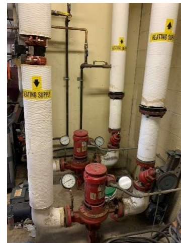
Office wing hot water pumps
