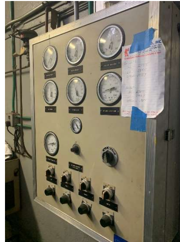
Main boiler room controls
