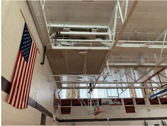
Gym AHU #1 (typ. 2 in this gym)
