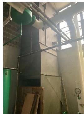
Main combustion air intake
