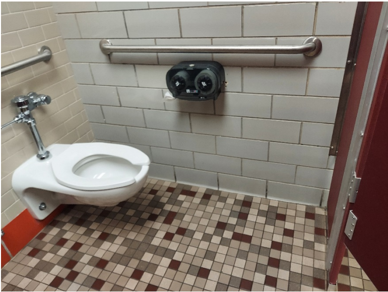
Toilet Room near Auditorium (Lack of 42" Clear in Front of Toilet)
