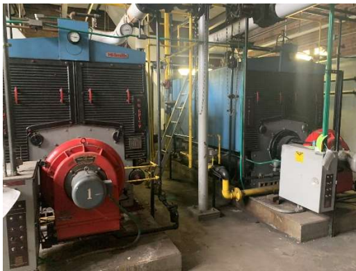
Main Heating hot water boilers
