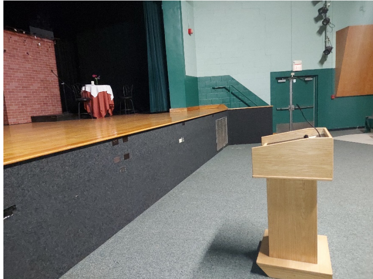
Auditorium Platform with no Accessible Route
