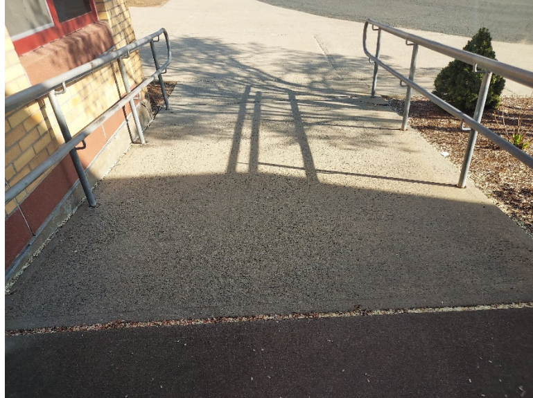
Cafeteria Door (Bottom of Ramp w/ Cross Slope Issues)
