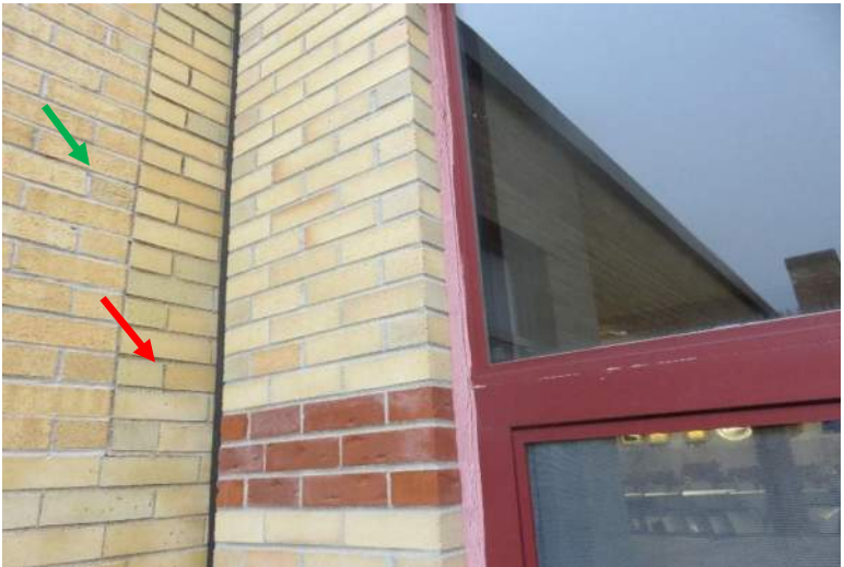
A unique perspective of building eras and types. The red windows and red brick occur in the 1995 construction. The brick on the lefthand side date to the original 1955 (green arrow) and 1979 (red arrow). Note the sealant failures.
