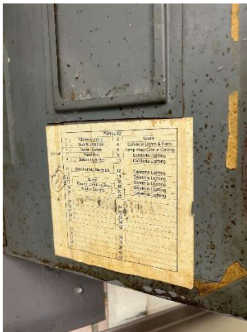
Corrosion on Panel K2
