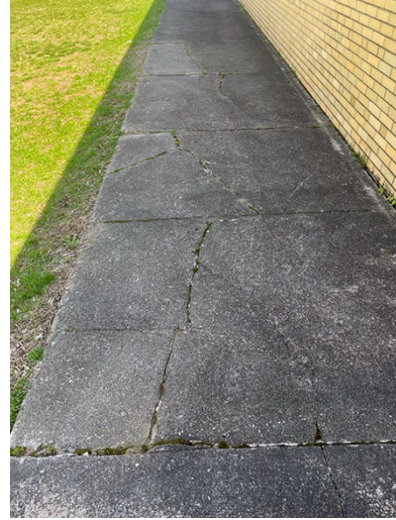
Image: Pedestrian pavement adjacent to the school building with numerous cracks.
