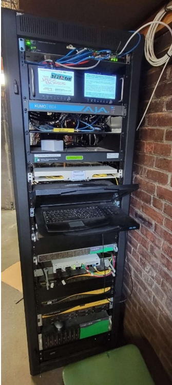
Community Cable Access Equipment Rack
