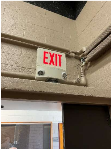
Emergency Battery Head
