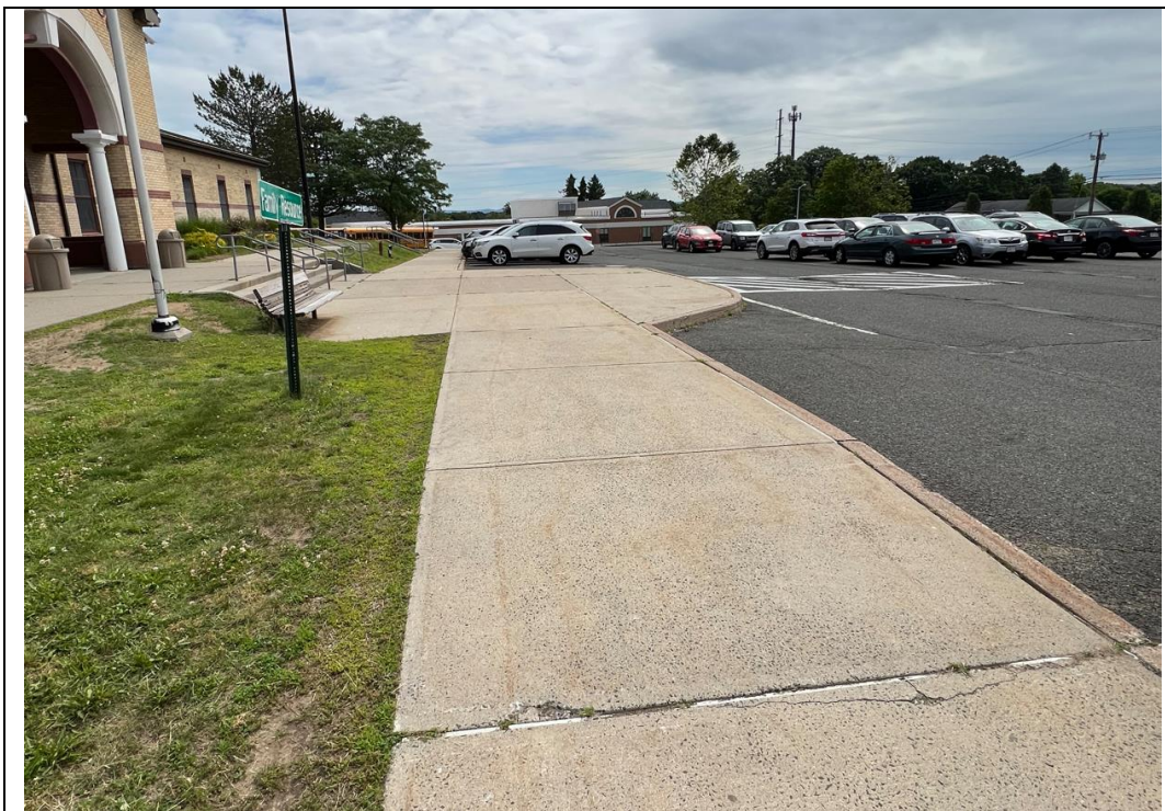
Figure 06: Typical condition of concrete walkways on the campus.
