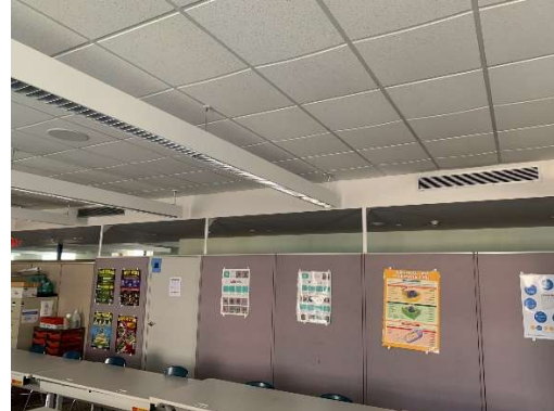
Sidewall supply diffuser
