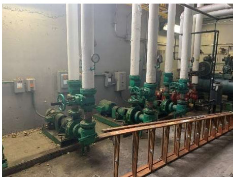
Main hot water pumps
