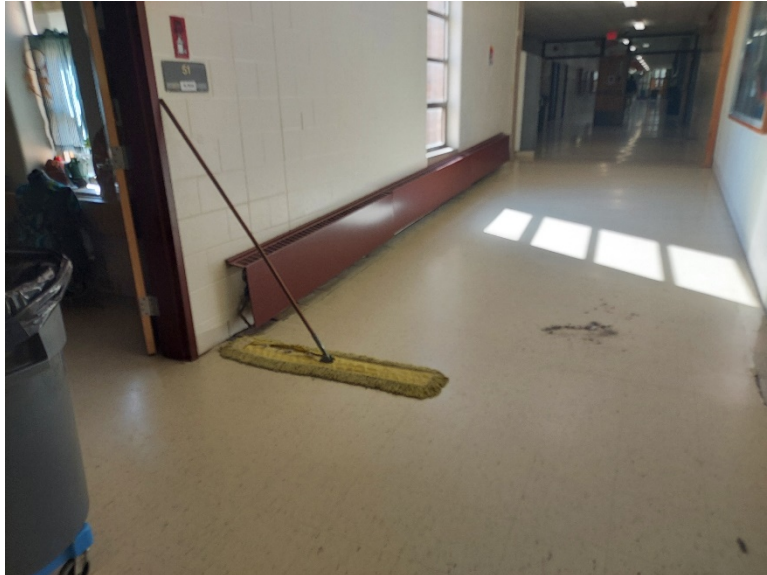
Ramp near Classroom 51 w/o Handrails
