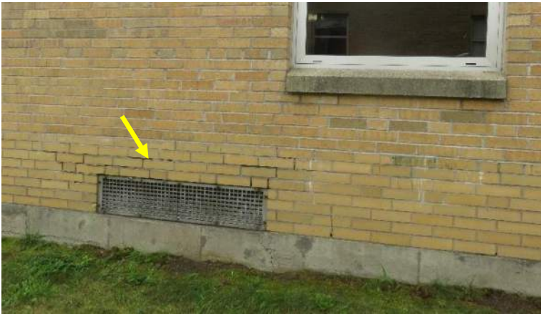
Deteriorated brick masonry conditions around unit ventilator. Also note staining of the masonry indicative of variant wall characteristics.
