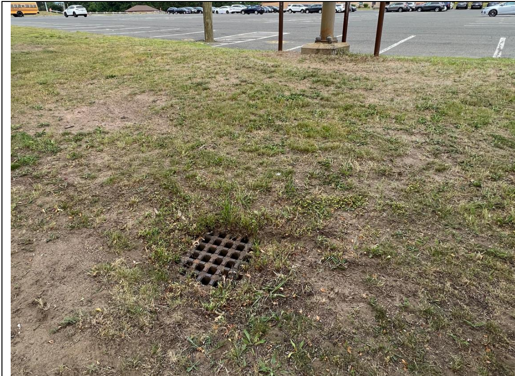
Figure 17: Overgrown catch basin drainage cover.
