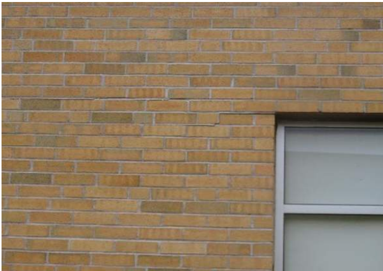
Masonry cracking in area of lintel. This may be related to 1979 masonry modifications.
