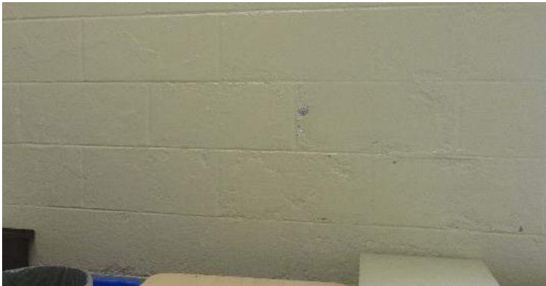
Excerpt of wall area where moisture related paint finish damages were observed.
