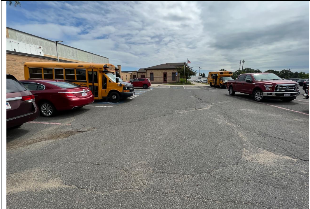
Figure 05: Longitudinal (Linear) and transverse cracking of bituminous paving in primary parking Lot.
