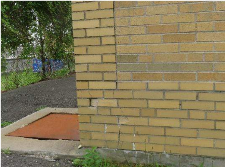
Detail view of damages at building corner. Note new 'yellow' brick added to the 1955 walls in 1979.
