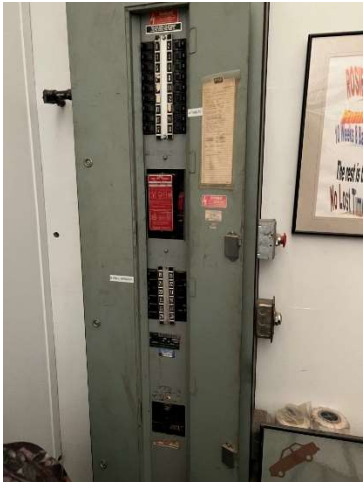
Electrical Shop Panel
