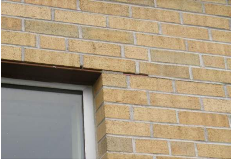
Detail view of typical lintel construction. Note minor mortar joint cracking from the dissimilar movement of materials.
