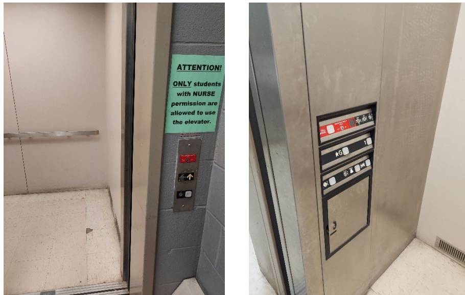
Elevator and Controls
