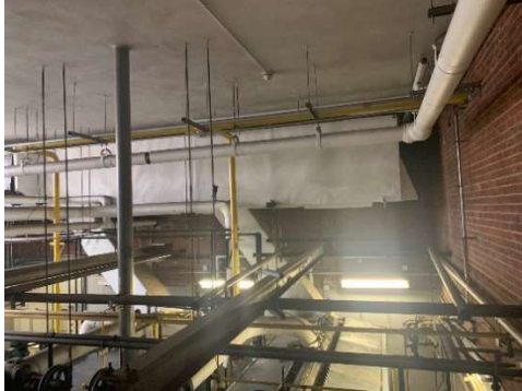
Main boiler flue exhaust
