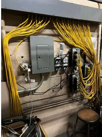
Stage Power Connections
