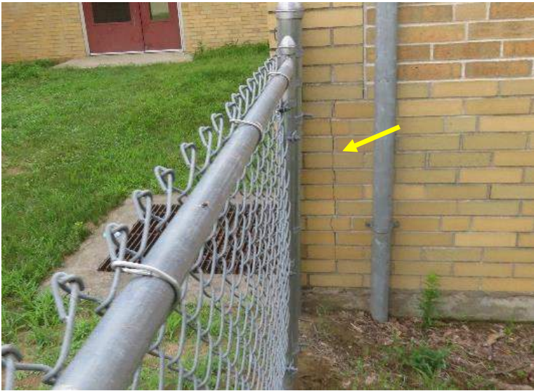
Cracking in masonry resulting from lack of control joints.
