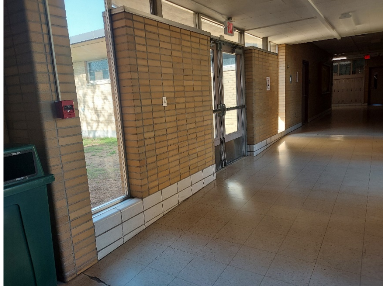
Ramp near Classroom 8 w/o Handrails
