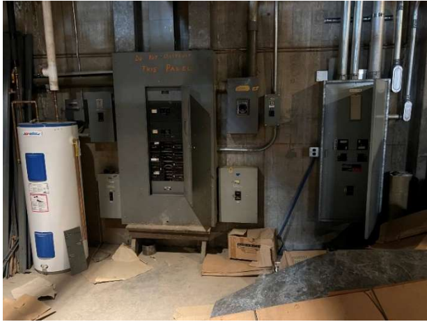
Maintenance Area Panels
