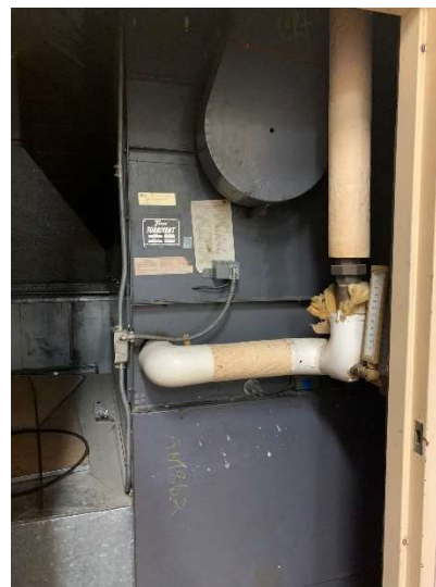
Original TORRIVENT cafeteria AHU
