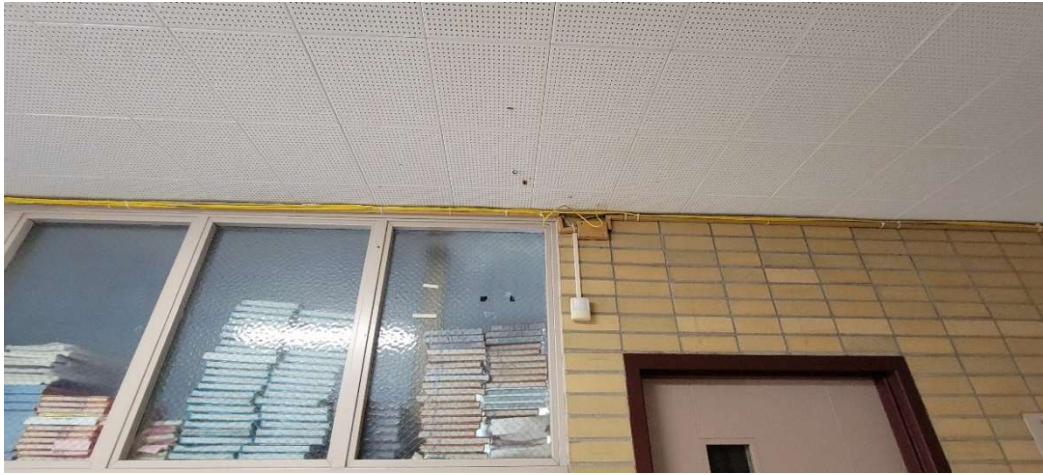
Exposed Cables in Hard Ceiling Hallway
