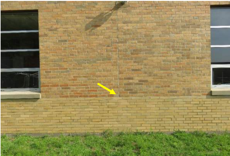
Detail view of original control joint location which was not carried through the newer work.
