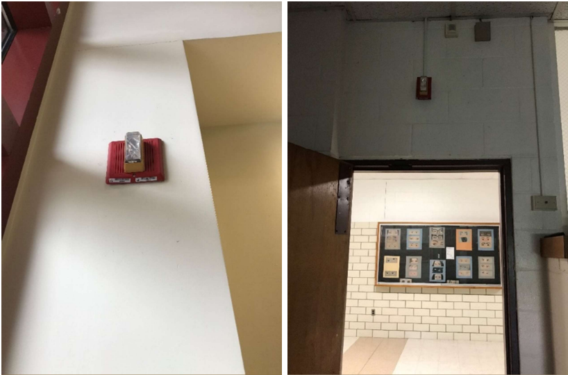
Building Notification Appliances
