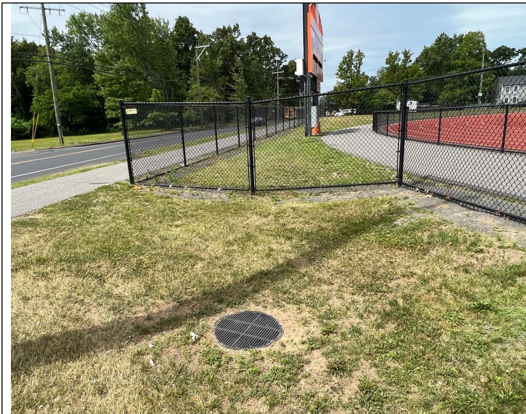
Figure 14: Typical condition of athletic facilities area drains
