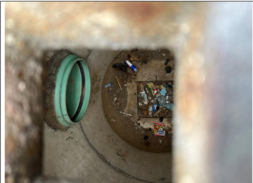
Figure 16: Catch basin with some debris and sediment.
