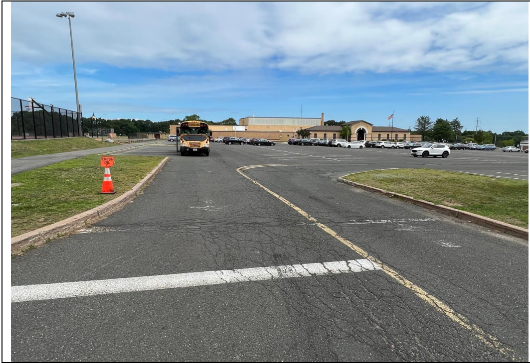
Figure 03: Typical condition of asphalt pavement on the campus, with alligator cracking visible.
