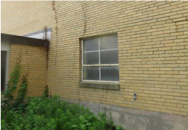
View of original steel framed window. Approximately 6 remain around the mechanical plant.
