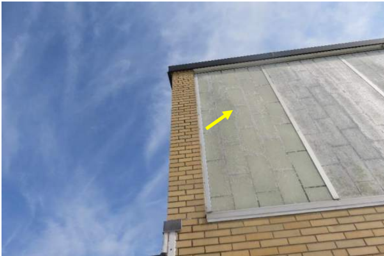
Detail view of deteriorated fiberglass panel conditions.
