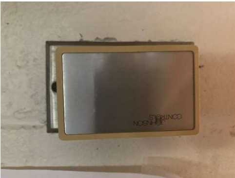
Typical classroom thermostat
