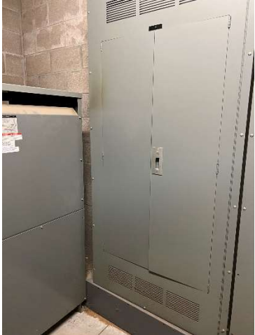
Electric Room Near Loading Dock
