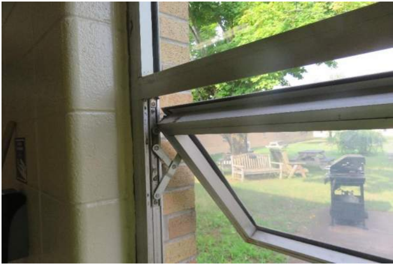
Yellow arrow notes compression gasket. It should also be noted that screens are not typically found on many of the window openings.
