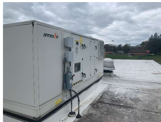
Locker room AHU (typ.2)
