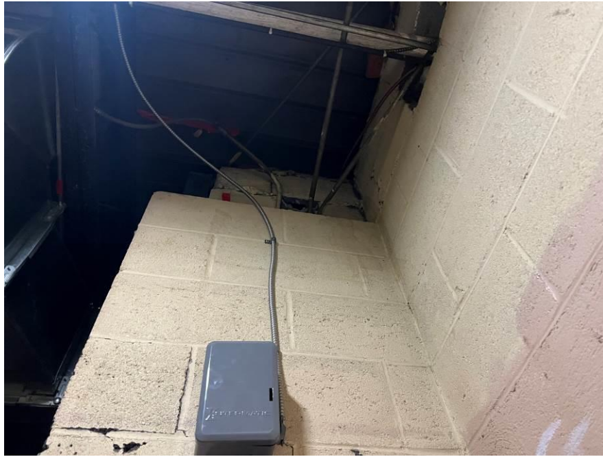
Example of minor cracks on interior masonry walls
