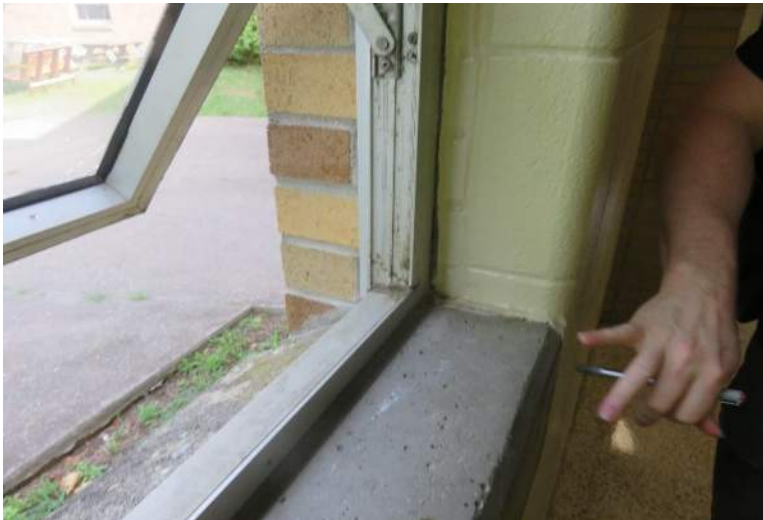
Detail view of typical awning sash construction. Note window sash rely on a single compression seal. Contemporary constructions, typically provide 2 or 3. Also note cast-in-place concrete sill, apparently installed as a repair in 1979.
