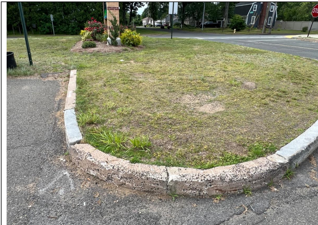
Figure 10: Typical condition of granite curbing on the campus, in most cases disjointed and in poor condition.
