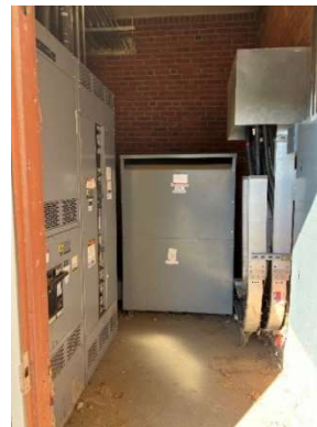
Main Electric Room
