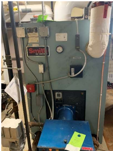
Office wing boiler
