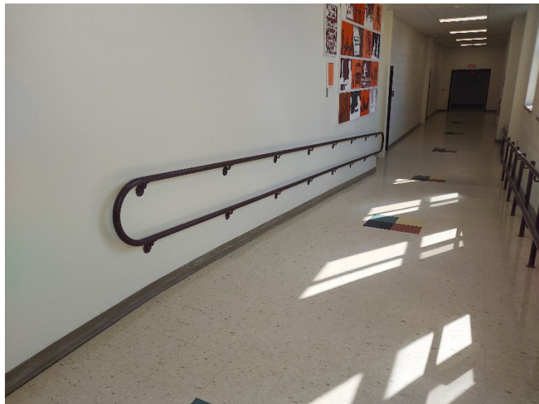
Ramp in Science Corridor w/o Handrail Extensions
