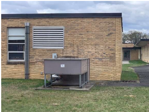
Air cooled condensing unit and louver
