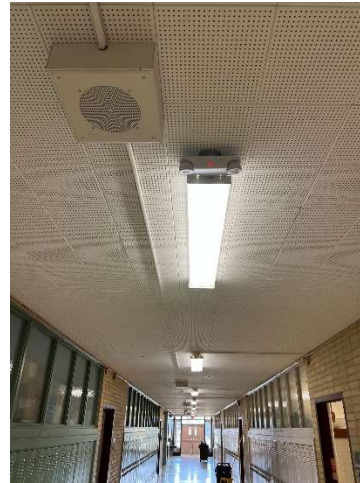
Hallway Emergency Lighting
