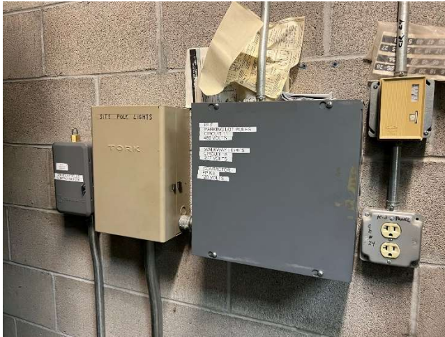
Exterior Lighting Controls
