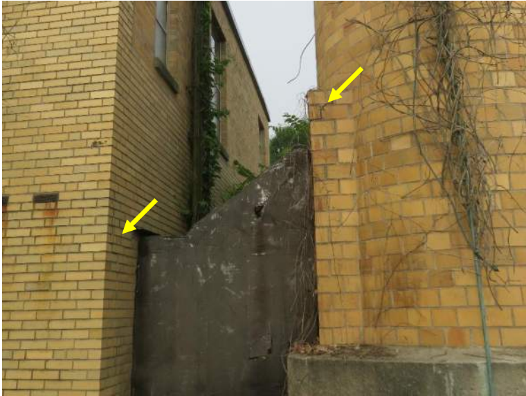
Detail view of deteriorated breach conditions. Masonry damages identified by arrows.
