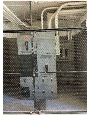
Original Electric Service
