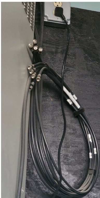
Abandoned Coaxial Cables (Old Security Cameras)
