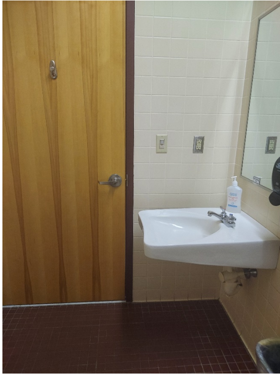
Family Services Toilet Room (Sink Obstructs Door Clearance)
