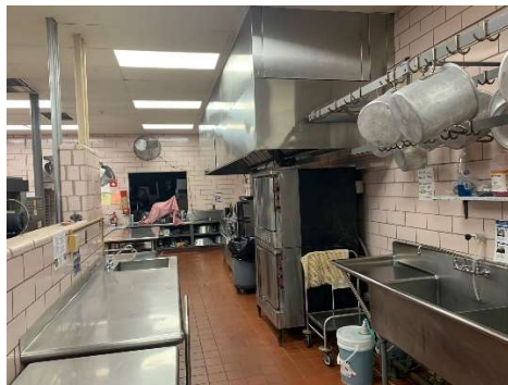
Kitchen Exhaust Hood
