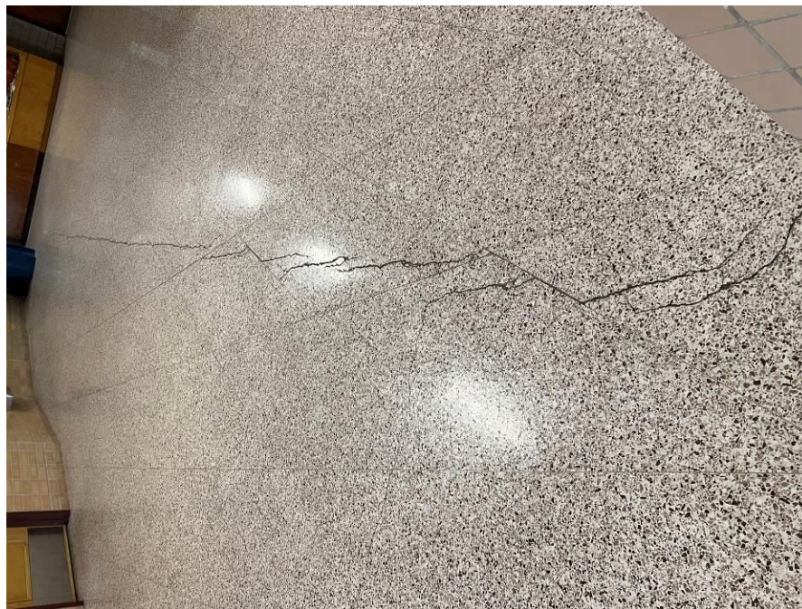
Example of cracks through the terrazzo flooring and the slab on grade
