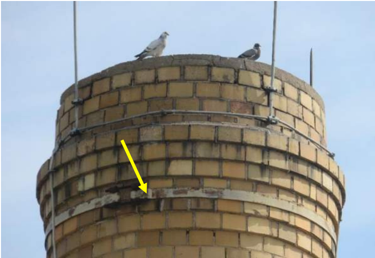
Note deteriorated concrete coping and mortar joints of chimney. Yellow arrow identifies previously applied compression band.
