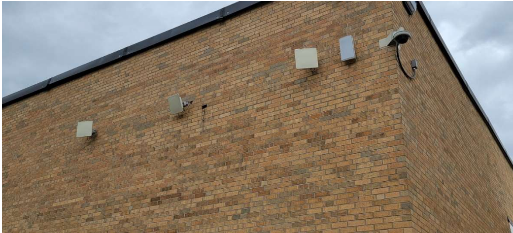
Exterior Mounted Point to Point Wireless Antennas to Stadium Press Box, Field House
