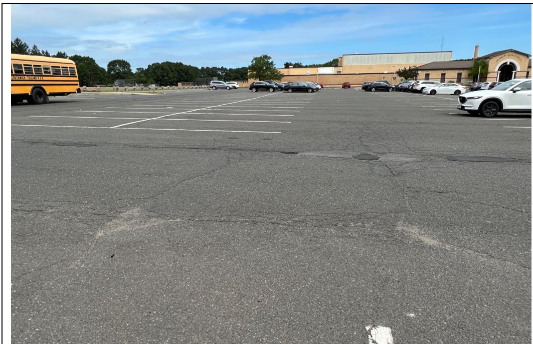
Figure 04: Longitudinal (Linear) and transverse cracking of bituminous paving in primary parking lot, with several patch areas also visible.
