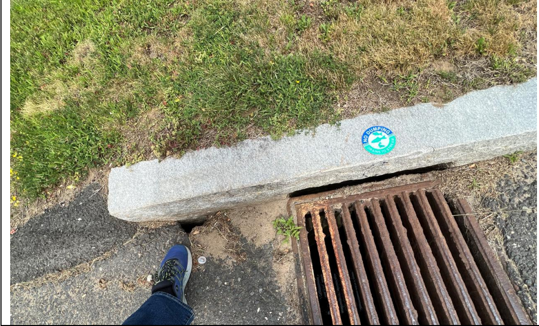
Figure 15: Small sinkhole observed at granite curb next to catch basin.
