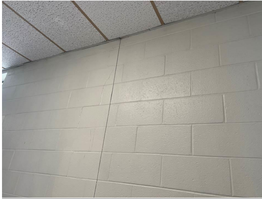
Example of cracks in interior masonry walls
