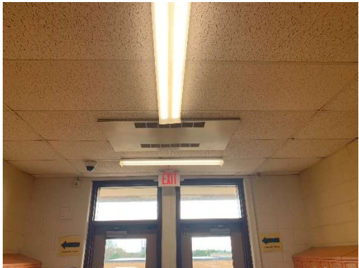
Unit heater by exit door
